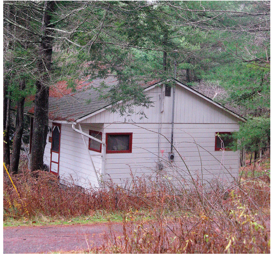
Located in the heart of the Luxton Lake community, this old cabin was shadowed by giant hemlocks and white pines, the gutters filled with decades worth of pine needles, and a rickety ramp was the only way approach the front door.
