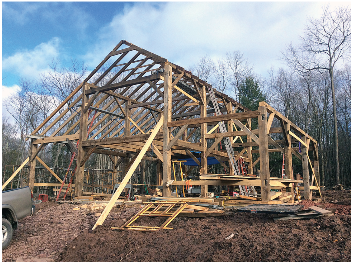
Using original beams, the frame of the barn is recreated on a new site.
